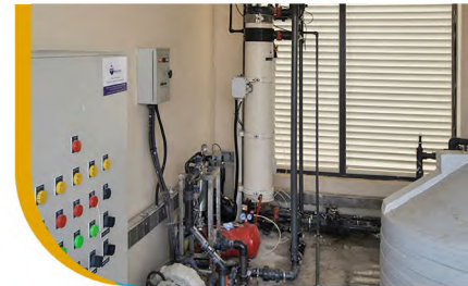
Grey Water Treatment Plant
