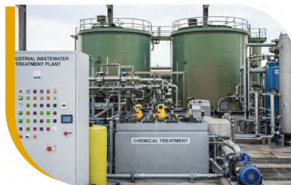
Industrial Wastewater Treatment Plant
