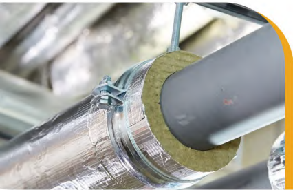
Exhaust Pipe Insulation
