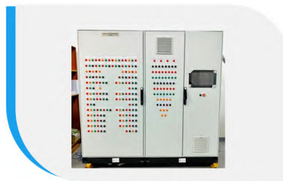
RO Plant control system
