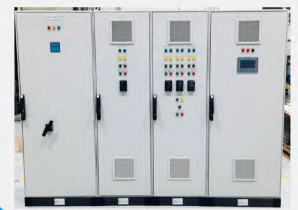
VFD & Soft Starters Panels
