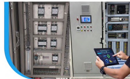
Standalone PLC/DDC system
