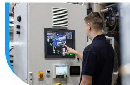
Boiler Control Panels
